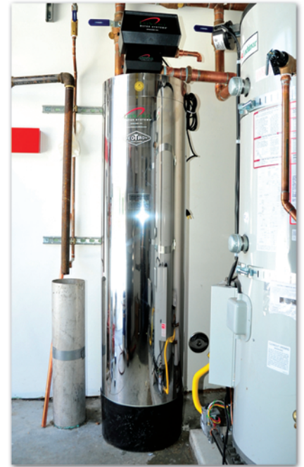
LifeSource System in the O.E. building
